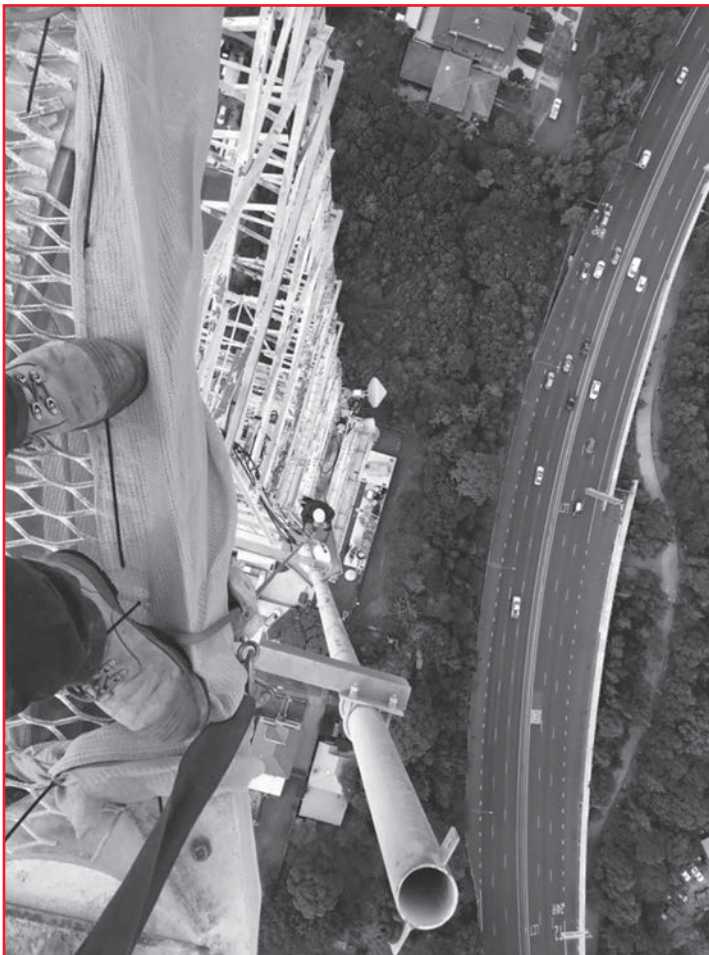
Figure 2 — Willoughby tower (with the Gore Hill freeway below). This illustrates the extreme heights at which telecommunications riggers work (Photograph taken by the study researcher).
