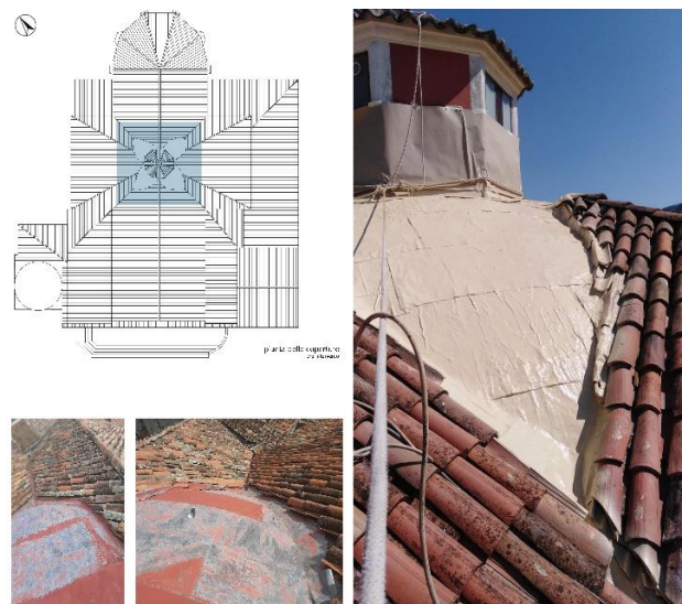
Figure 8. Situation at the extrados of the dome. It is possible to clearly see the 4 areas without waterproofing.
