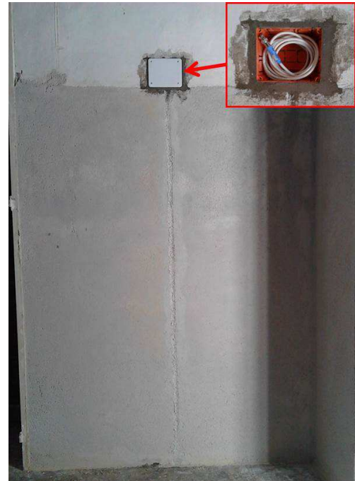
Fig. 5. Picture after the installation of the SE is completed. The inset shows how the coaxial cable is rolled up and placed inside the wall box.
