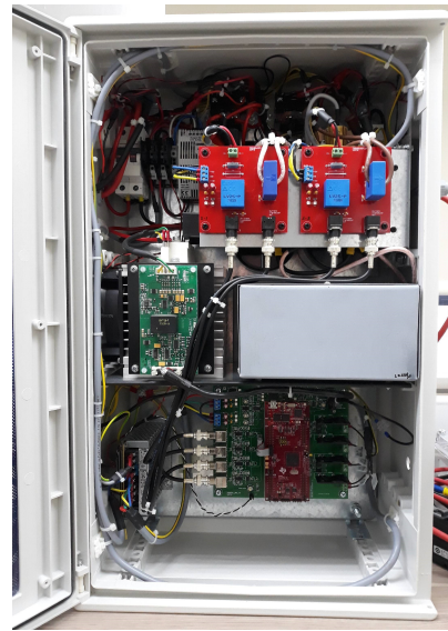
Figure 2: A microgrid DC-to-DC converter implemented for the DC microgrid in the IEPC labs.
