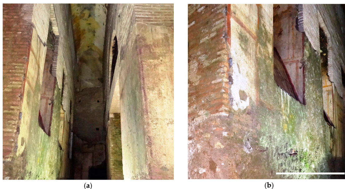
Figure 2. Two different views of the sampling site in Room 93 with the evident phototrophic biofilms causing discolouration of the walls. (a) front view of the corridor present in Room 93; (b) detailed image of the wall object of the investigation with the evident presence of the green biofilm; scale bar = 2 m.
