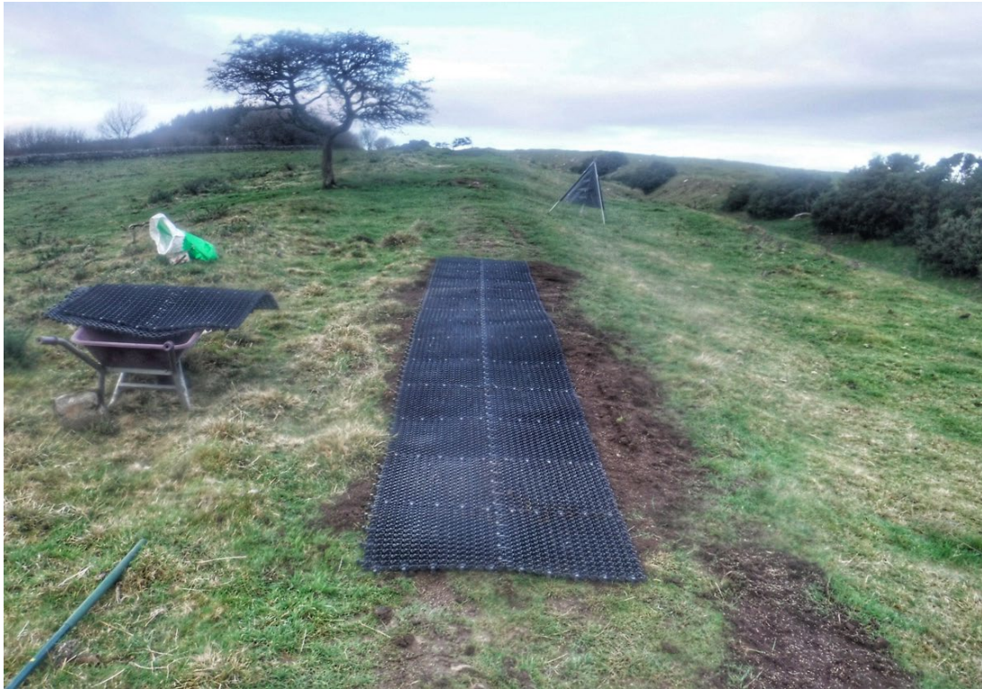
Figure 13: A flexible membrane covers the repair to allow the new grass/root system to become established. © Northumberland National Park
