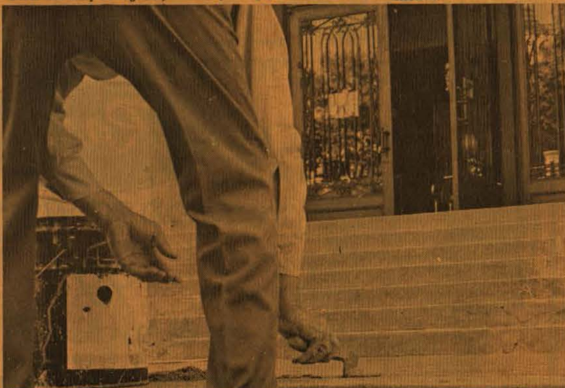
SEPTEMBER IS NOT ONLY the time for repairing minds but the time for repairing cracks in the steps of the library. This university workmen are repairing cracks in the rear steps of the 40 year old building.
