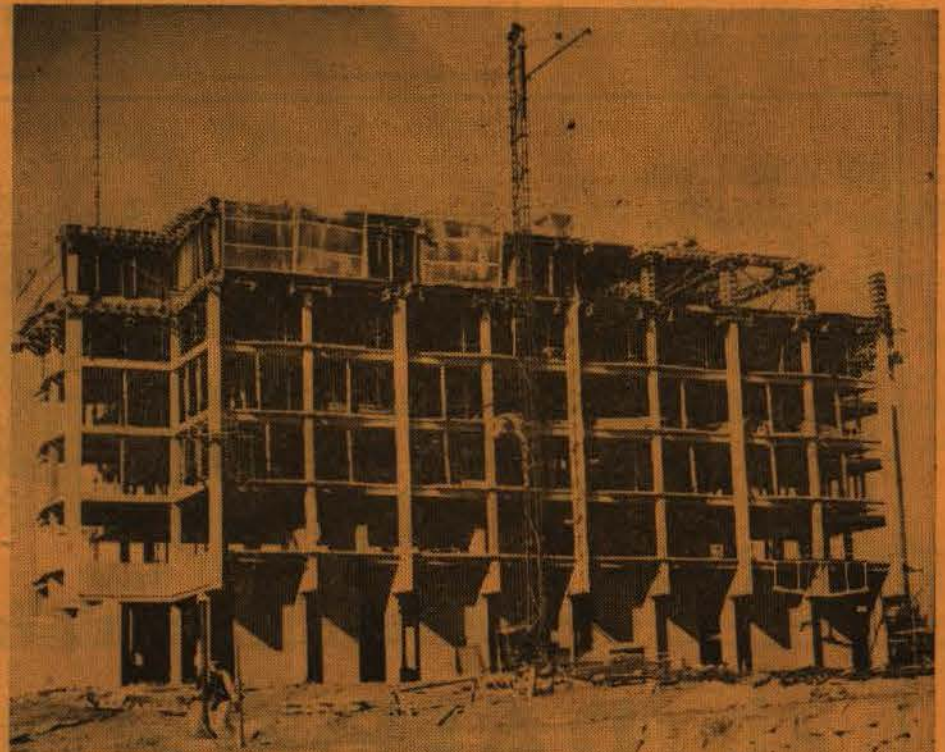
industrial arts departments. The building will be made up of two four-story wings connected by a one-story section which will adjoin the Industrial Arts Build-
