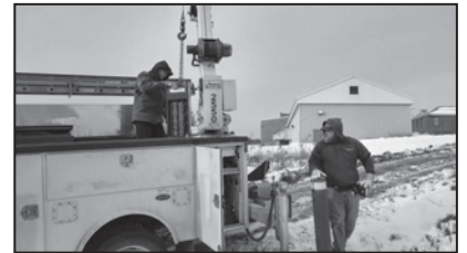
A crew from Stevens Electric (Monmouth, ME) prepares to unload a new Muffin Monster hydraulic grinder unit at Pump Station 2, behind the Bolduc Correctional Facility in South Warren. December 14, 2017
