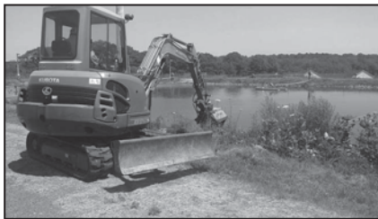
Joel Wentworth of Union mows weeds on the bank of our primary lagoon using an excavator-mounted flail mower. July 19, 2017.
