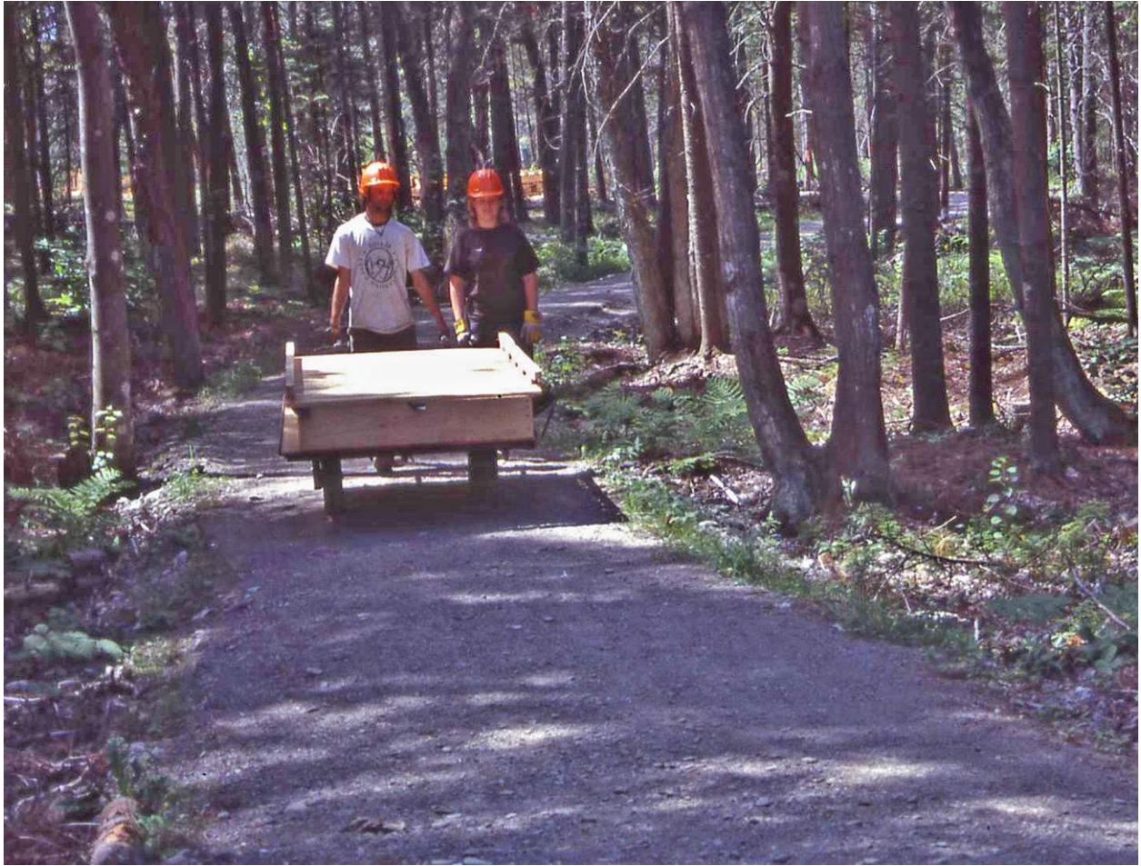
Fig. 13. Transporting a boardwalk section on a special cart along the trail from the assembly site to the incomplete boardwalk. Ronald B. Davis photo.
