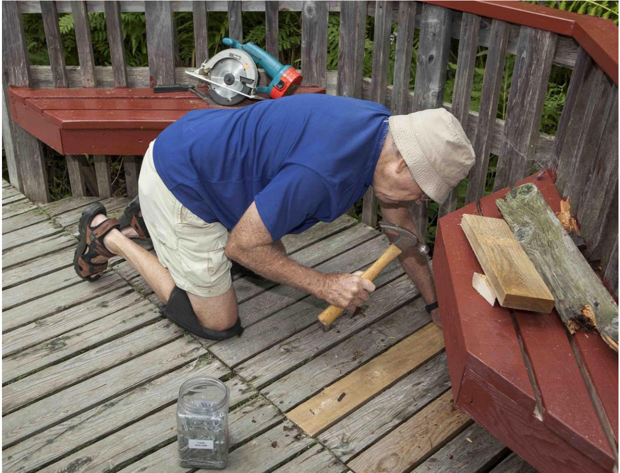
Fig. 30. Phil Locke replacing a broken deck board at IS1 on 13 August 2012. Ronald B. Davis photo.
