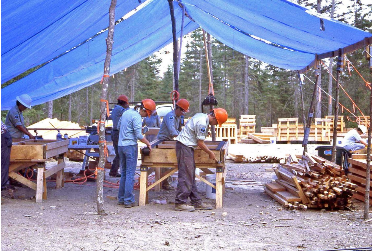
Fig. 15. Maine Conservation Corp crew members at assembly site in summer 2002. Member in central foreground is spiking an end joist on a boardwalk section (see Fig. 6) using a small sledgehammer (zoom in). The incomplete section rests in a jig supported on sawhorses. An incomplete section in another jig is at far left. Its middle joist is in place. The heads of three spikes can be seen on the end joist (zoom in). A pile of bump railings is on the right. Stockpiled components of interpretive stations including railings (see Fig. 8) occupy right background, and a pile of large dimension lumber rests in far-left background. Ronald B. Davis photo.
