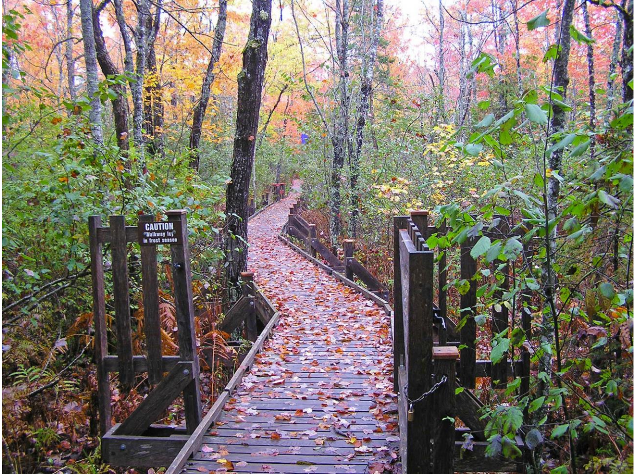
Fig. 29. Boardwalk gate chained in open position in early October 2012. Note that the first ~120 ft (~37 m) of the walkway to IS1 (red railing and bench barely visible) is supported by pilings. The original floats were replaced by pilings in April 2006. 32 Ronald B. Davis photo.
