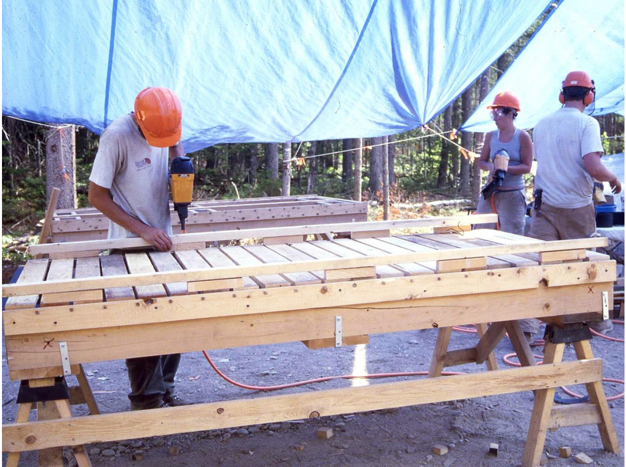
Fig. 17. Final stage of assembly of a boardwalk section in the jig in the foreground. An MCC member is nail-gunning a bump railing atop riser blocks at the ends of the deck boards. On the closest face of jig, the insertions of the half-inch diameter pegs used to space apart the deck boards can be seen. The jig in the background contains a section's longitudinal joists with end joist attached on the right, with the left end joist leaning against the jig. Ronald B. Davis photo.
