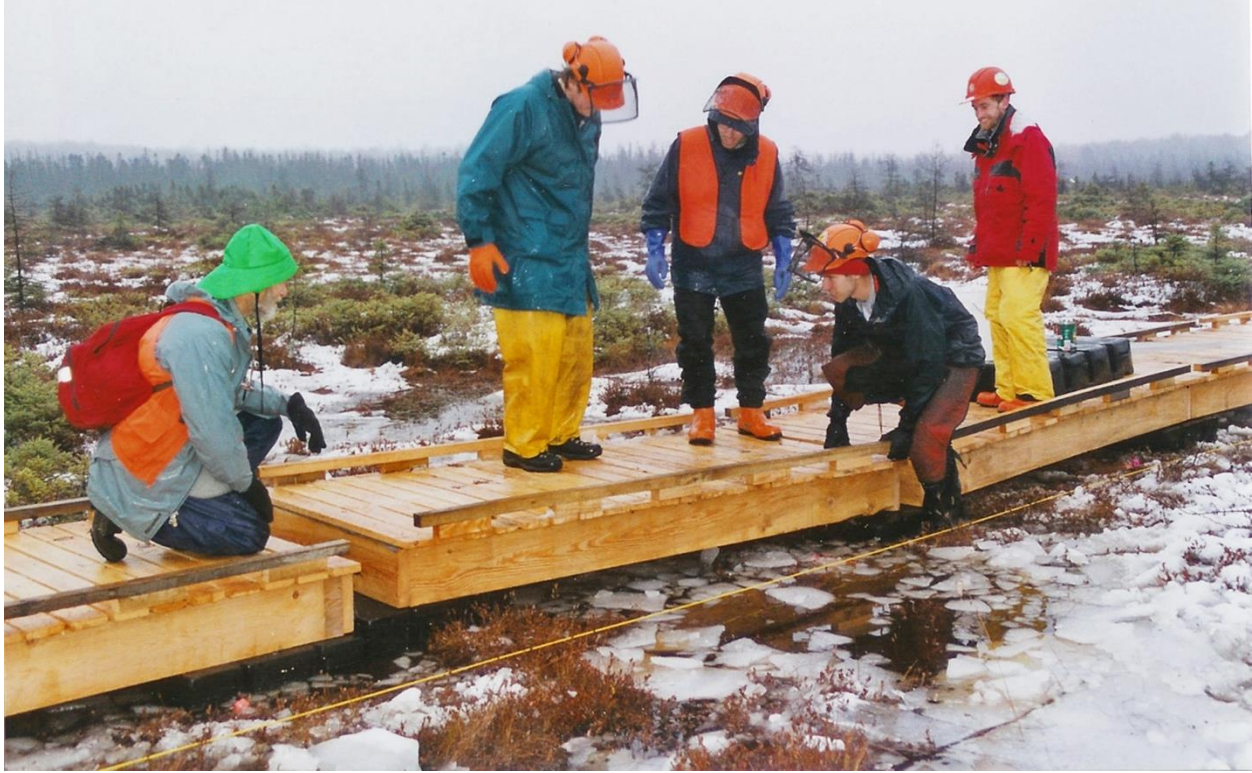
Fig. 22. Remaining members of the MCC-leader teams adjusting the last-emplaced of 509 boardwalk sections while Ron Davis (green hat) looks on. 93 The photo was taken shortly after the two arms of the boardwalk loop were joined at the middle of the open bog at 2 PM on 22 November 2002. Despite being a cold, wet and dreary day, our hearts were warmed by the “drive the golden spike” occasion. The remaining gap of about a 1 ft (~0.3 m) would be easy to bridge when work resumed in spring 2003. Author Ron Davis in green hat observes the four MCC leaders. Photographer unknown.
