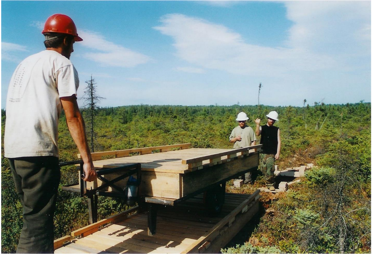
Fig. 19. Arriving with a section at end of incomplete boardwalk. The pair of MCC members in the bog have prepared footings for supporting the arrived section. Ron Lisnet UM photo.
