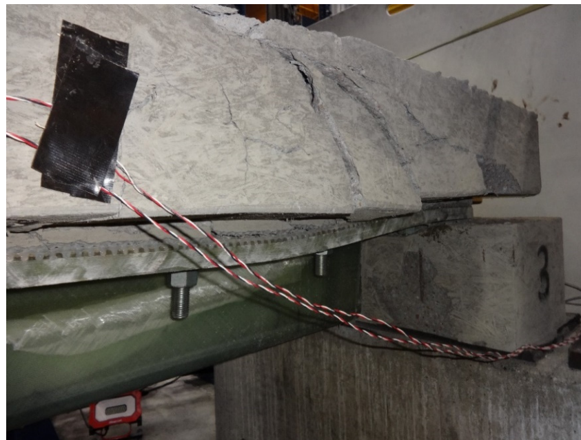
Figure 15. Post-Failure Image of Beam B1.
