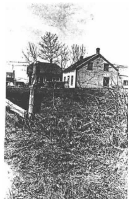
Mama's house when it was being demolished. Uncle Freddie's house behind it.
