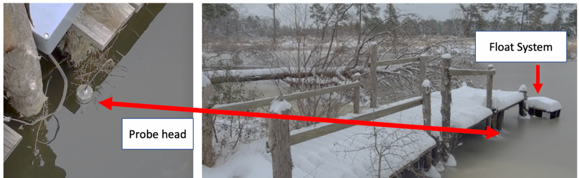
Figure 16: Field deployment of the HyLO-Mo System
