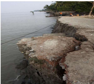
Figure 11: River erosion, Lalmohon Bhola
