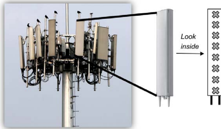
Figure 5.1: Base Station Tower with Sector Panel Antennas. An array of elements is shown in the interior of one panel antenna. Picture extracted from [1].
