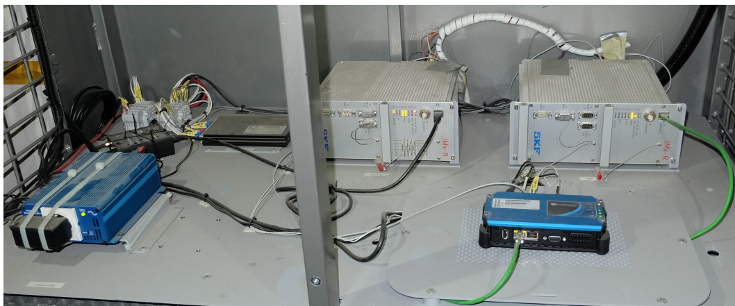
FIGURE 7 Location of the acquisition system
