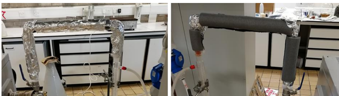
Figure 4-28: Sleeve, the inner second thermal isolation layer on top of mineral wool (right), third layer of isolation, aluminium tape (left)
