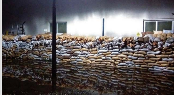
Sandbags at Lancaster substation
