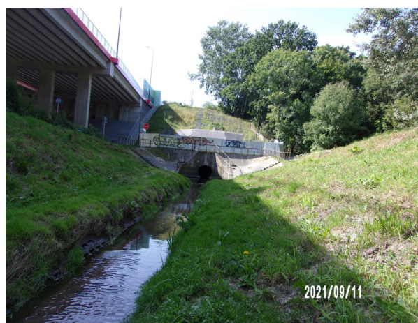
Figure A7. A view of the outflow from Ursynów rain collector measuring 4 metres in diameter, with a flow of 8 \text{ m}^3\text{s}^{-1} (source: own).
