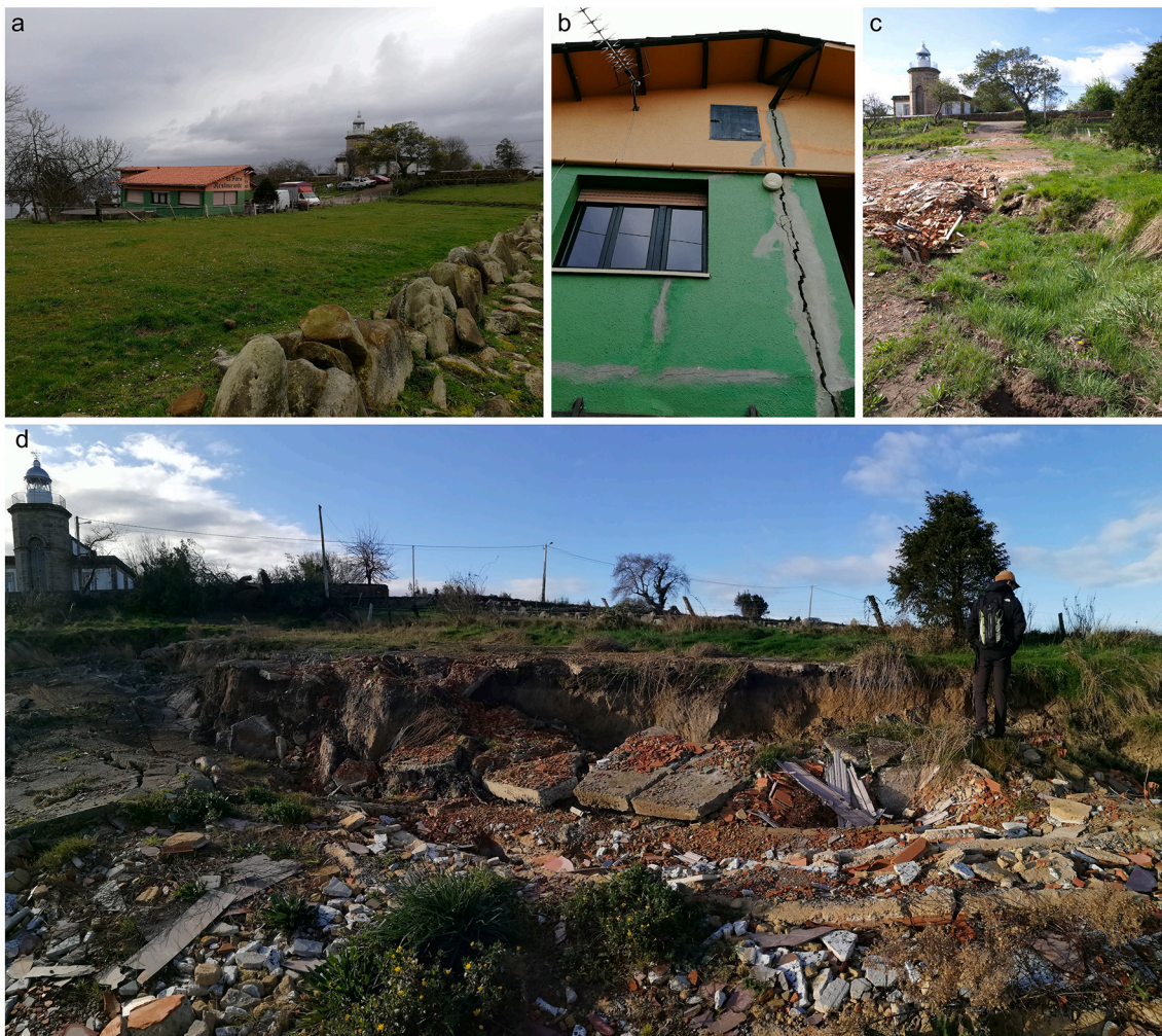
Fig. 2. a. View of the Tazones Lighthouse surroundings at the time of the restaurant eviction on February 20th 2018, after the critical enlargement of the cracks. b. Detailed view of the cracks in the restaurant building at the date of eviction. The eversion of cement in the wall shows the attempt to repair old cracks that had developed before. c. d. Two views showing the evolution of surface cracks in the Tazones Lighthouse area on April 26th 2019 and January 17th 2020, respectively.
