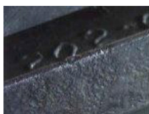
FIGURE 6. Rough Damage (Khode 2019)
