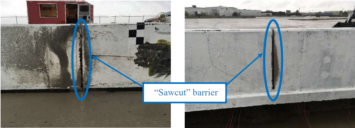
Figure 14: Inside (left) and Outside (right) Face of Barrier after Concrete Barrier (D3) (Akintunde et al. 2021)
