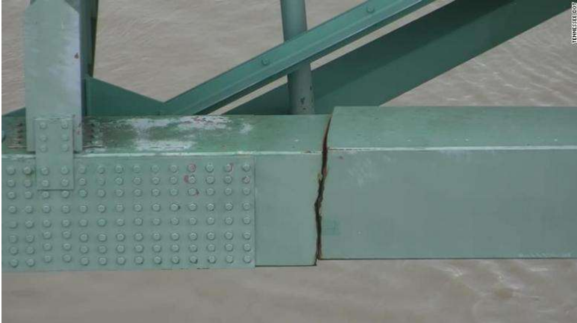
Figure 3: Full Height Crack on Bottom Chord of Hernando DeSoto Bridge
