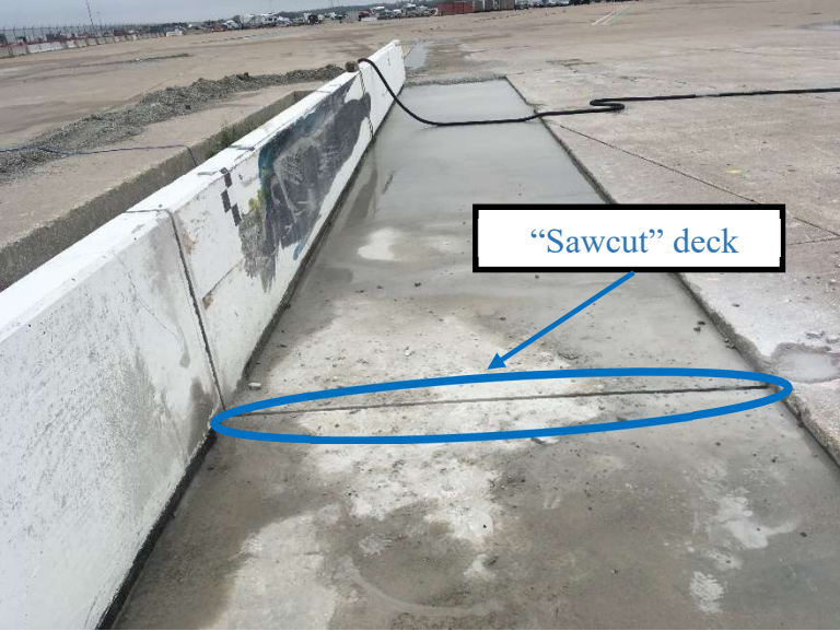
Figure 15: Deck Damage (D3) (Akintunde et al. 2021)
