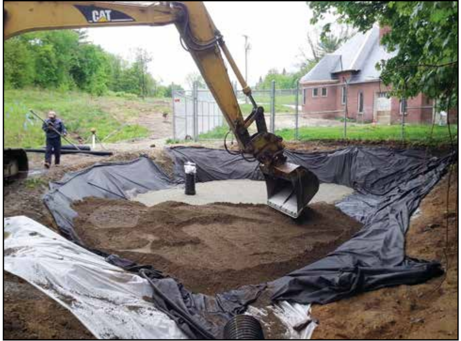
Installation of a bioretention system next to the City’s historic 1888 water works pumping station.
