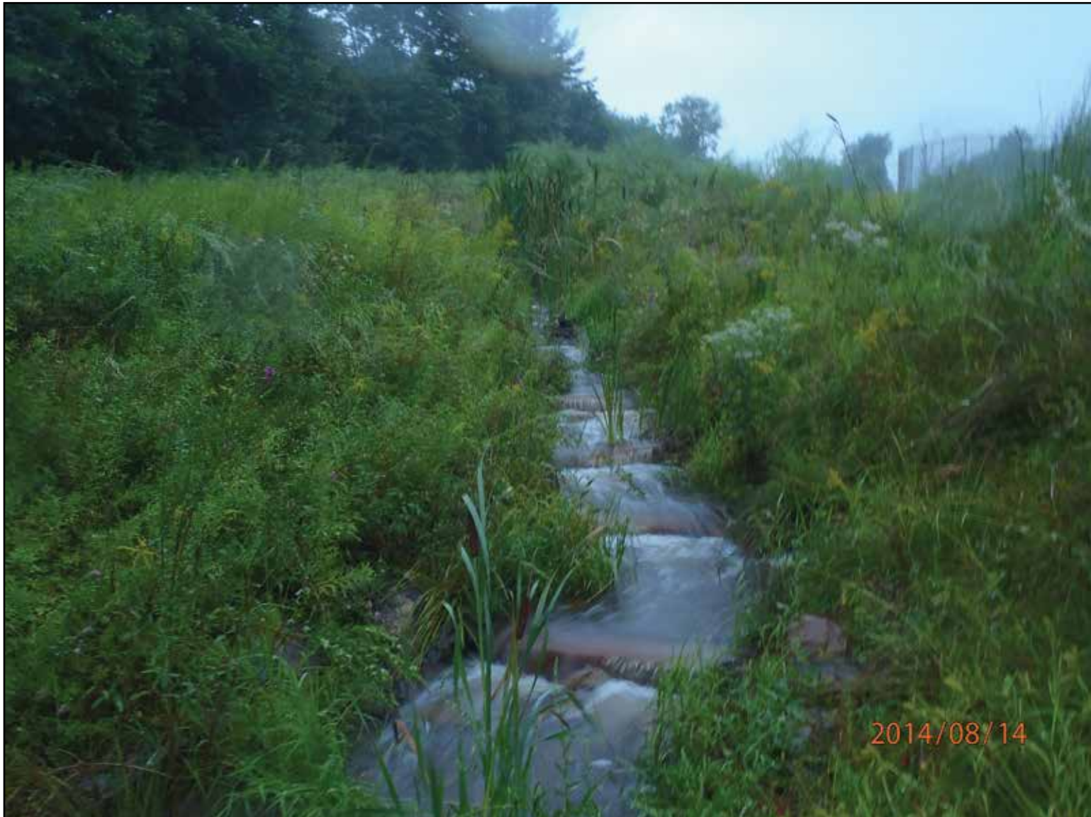
A step pool sequence along an 1,100 ft long section of a day-lighted and restored stream.
