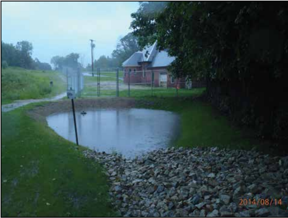
Installation of a bioretention system next to the City's historic 1888 water works pumping station.
