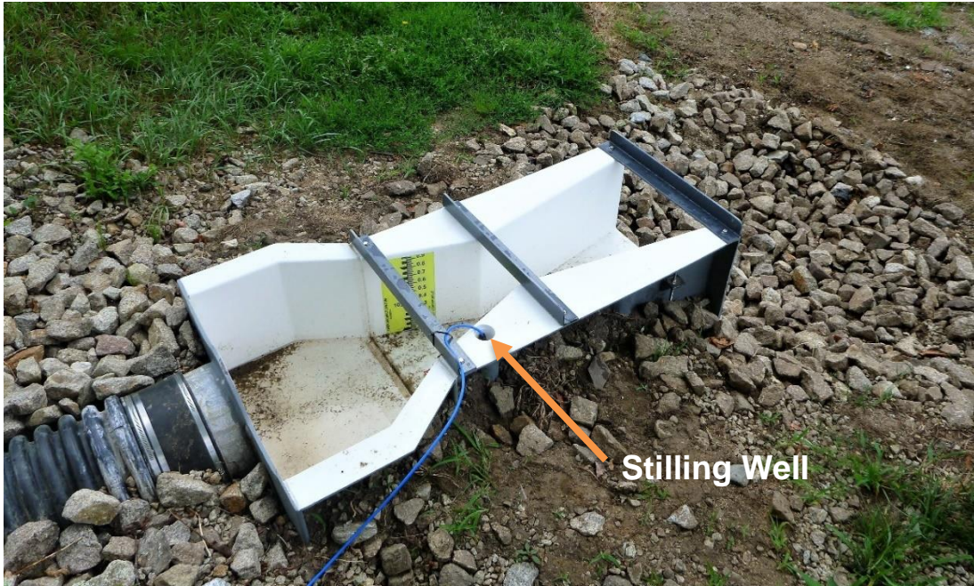
Figure 14: Inlet monitoring using an OCF 36x8 inch Cutthroat Flume. The blue line seen at the bottom center of the image is the data line for the pressure transducer located in the stilling well.
