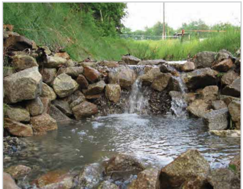
In April 2007 the filter berm swale failed after a torrential storm in which the swale conveyed a 6.8 cfs peak flow (more than six times the design flow).
