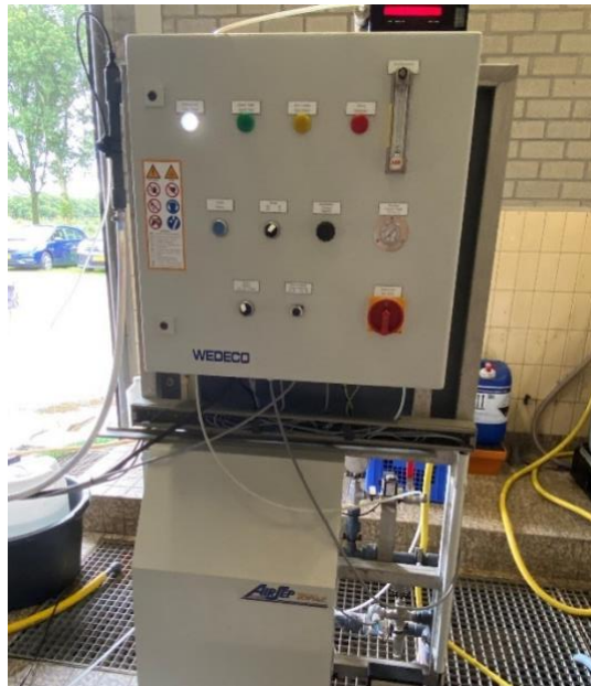
Figure 13: The back of the ozone generator with the electrical controls.
