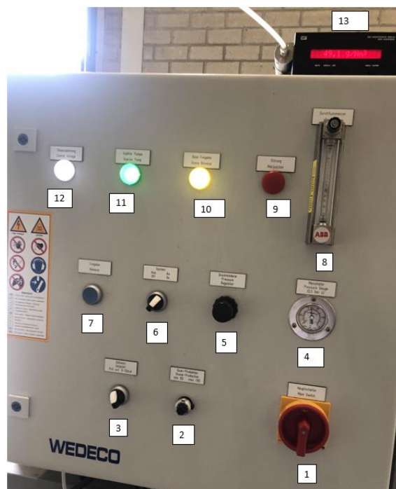
Figure 53: The back control panel on the ozone generator in the CO.4 pilot.
