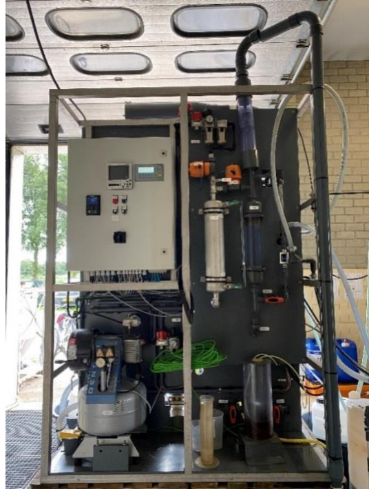
Figure 11: The back of the pilot plant that houses the electrical controls.
