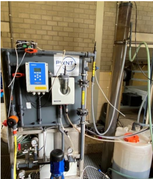
Figure 12: The front of the ozone generator with the bubble column in the background.
