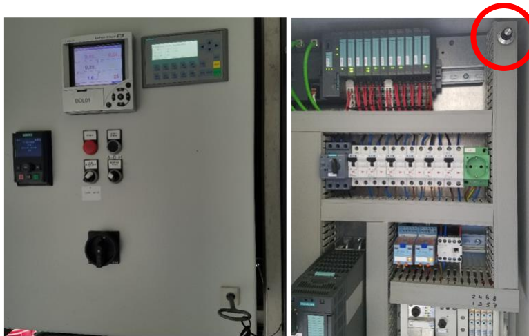
Figure 54: The interior and exterior of the pilot's control panel.
