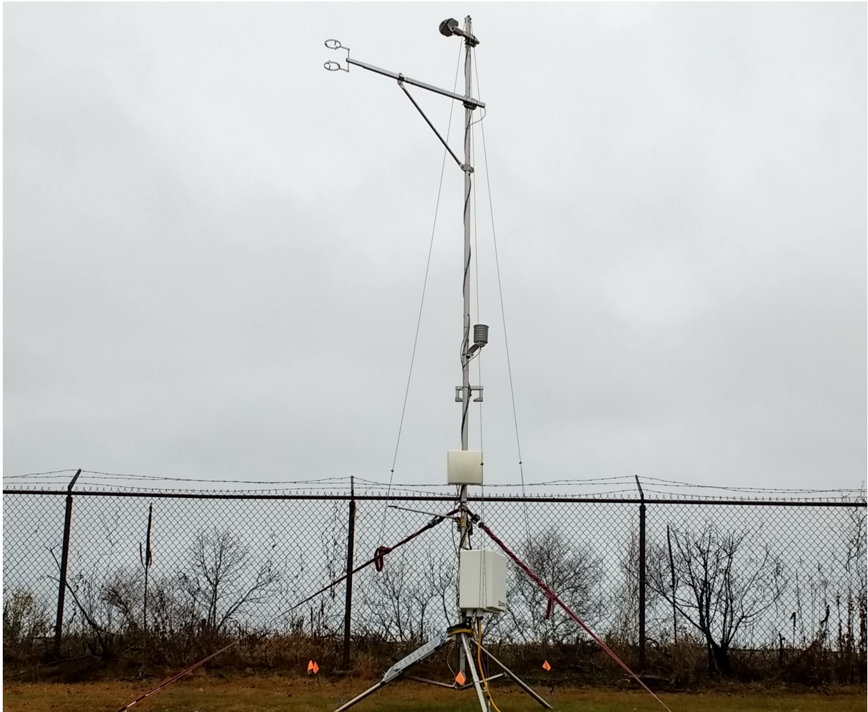
Figure 3.2. Weather station installed in Newcastle, NH.
