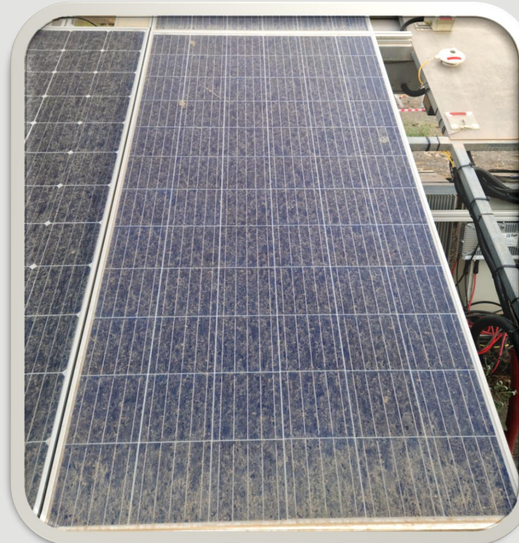
Fig. 1 Soiled PV panel
