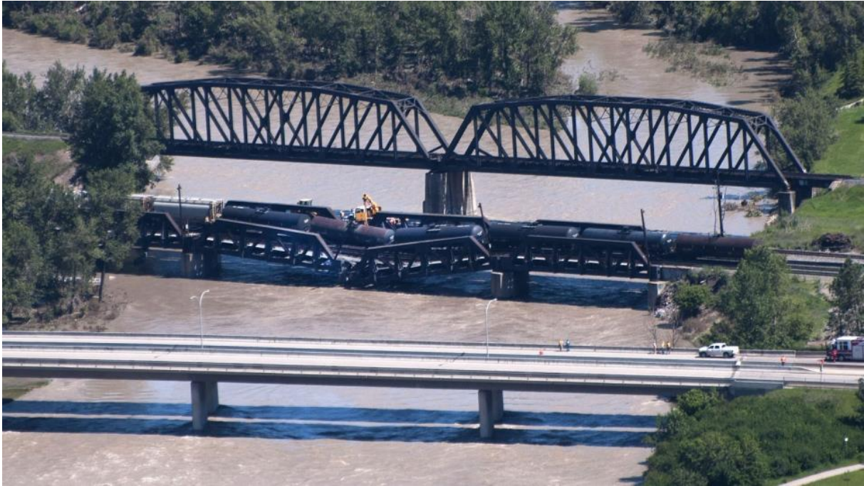
Figure 1.1: Scour-related bridge failure in Alberta, Canada (CTV News, 2013)
