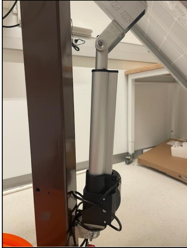
Figure 6: Close-up view of the N-S linear actuator attached directly to the upright post. This linear actuator is responsible for movement along the N-S axis of rotation.
