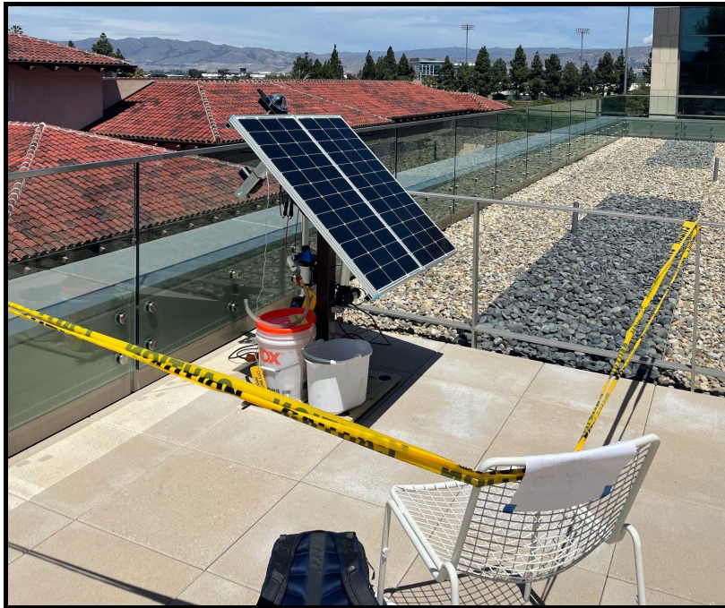
Figure 35: Solar tracker test setup for two 24 hour tests. Tests conducted on 5/8/2022 and 5/9/2022 on Santa Clara University campus.
