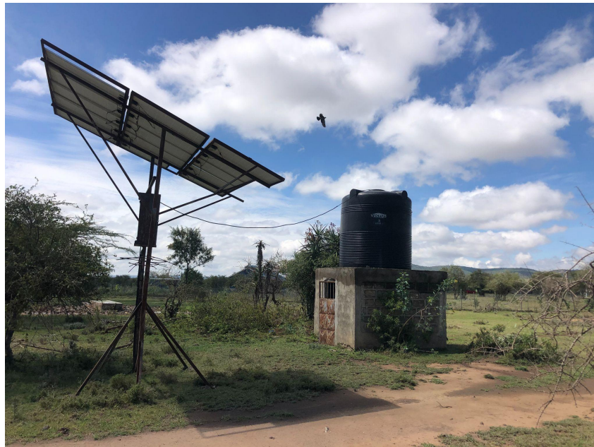
Figure 1. Supetai Well and solar power pump system.
