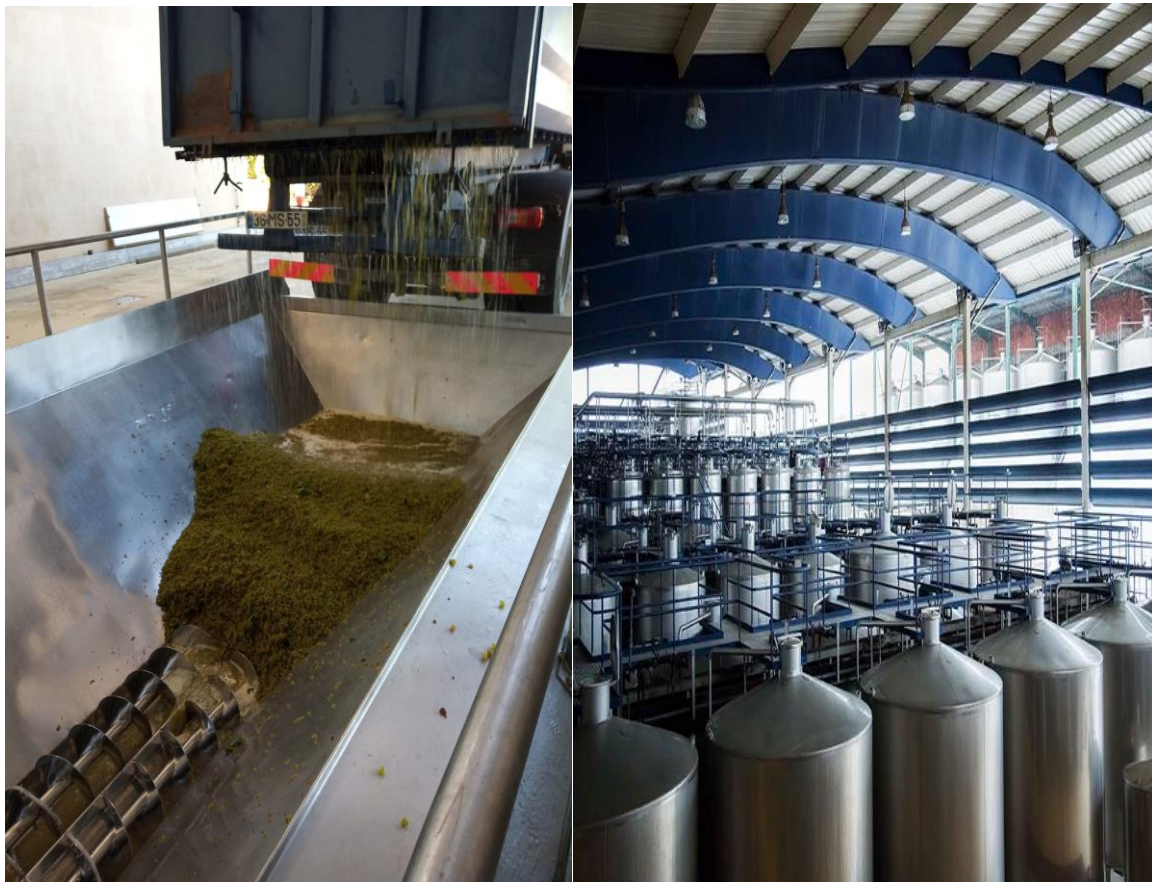
Figure 12: Conveyor and Cellar(Roy)
