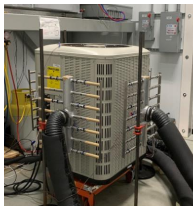
Figure 3: Outdoor Unit Connected to Air Sampling Trees
