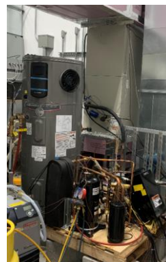
Figure 4: Indoor Air Handler, Compressor, Suction Line Accumulator, Brazed Plate Heat Exchanger, and 50-gallon Water Tank
