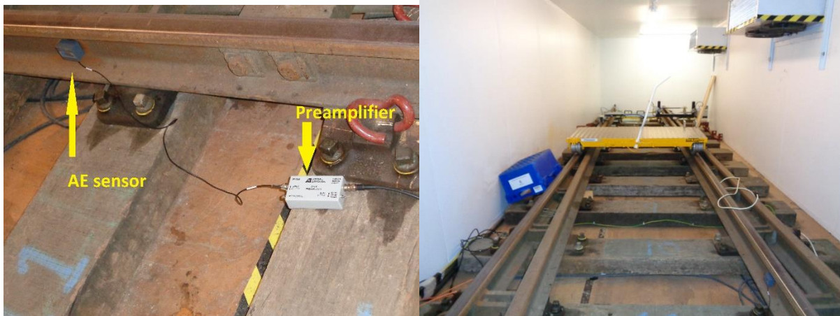
Figure 0-0-0-9: Wayside installations (left figure) and motorized trolley (right figure)
