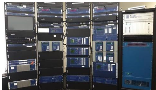
Figure 1: Protective Devices and RTDS
