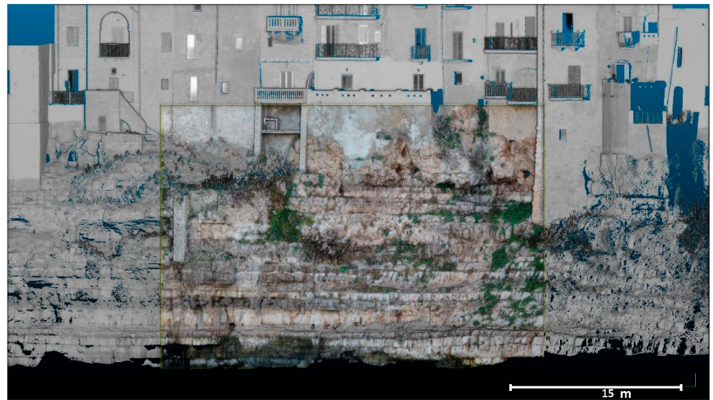
Figure 4. Final high-resolution point cloud (RGB colors) of the study site obtained by means of UAV technique and aligned on a georeferenced TLS point cloud (in gray) to avoid doming deformations. The UAV point cloud has a surface density of 13391 points/m 2 , corresponding to a mean point spacing of 9 mm.
