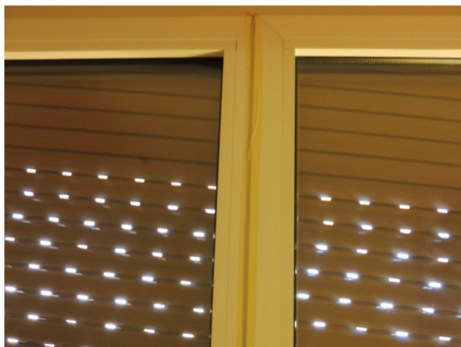
Fig. 1. Detail of scotch tape around window.
