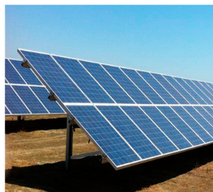
a) Fixed-tilt PV installation
