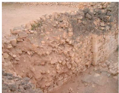
Collapse of external layer
