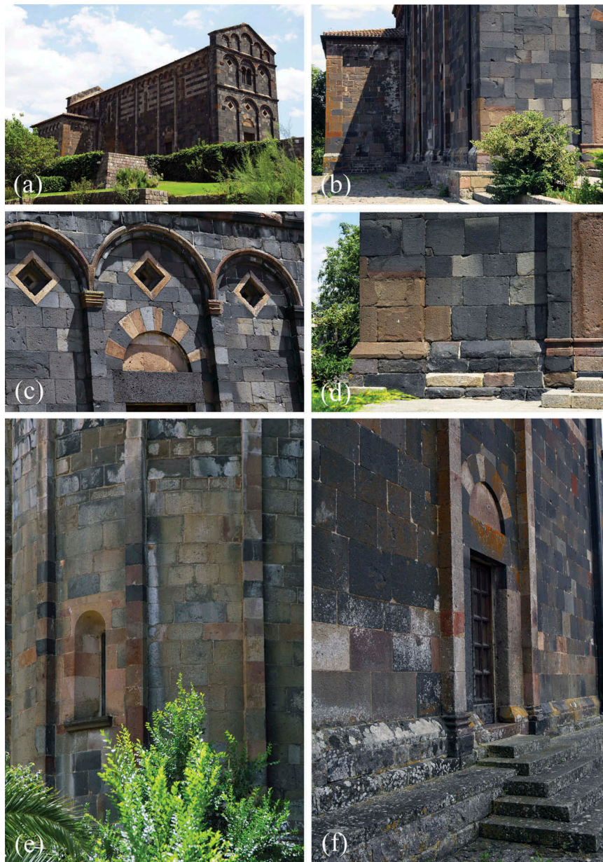
Figure 2. The San Nicola Church: (a) South-West side overview; (b) South side of the façade overview and Western transept of the Church, where upper and middle parts are covered by whitish patinas; (c) details of the three arches in the front door of the Church, where whitish patinas occur under the horizontal cornice; (d) basal plinth of the main façade, where important processes of exfoliation and flaking occur, causing detachment of flakes up to 2 cm thick; (e) the apse view, with presence of whitish patinas (at the top) and beige/ochre fouling (in the middle and lower parts); and (f) the Western side of the Church, with presence of whitish patinas and organic films (mainly lichens) in the low plinth and in some ashlar.
