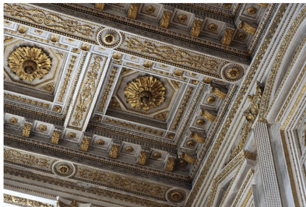
Figure 6: Photograph of the coffers as visible from the nave interior; the lower load-bearing beams are covered with decoration; the metal wire ends with the decorated circular button visible beneath the beams.
