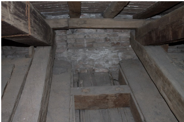
Figure 3: Photograph of the coupled trusses insertion in the perimetral walls and the shorter span between them; the upper part of the smaller structural shelves is visible.
