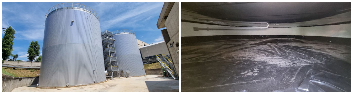
Fig. 6. Left: TESs in ‘Centrale Nord’, Brescia, Italy. Construction timelapse video available online [22]. Right: protective membrane installed in ‘East’ TES.
