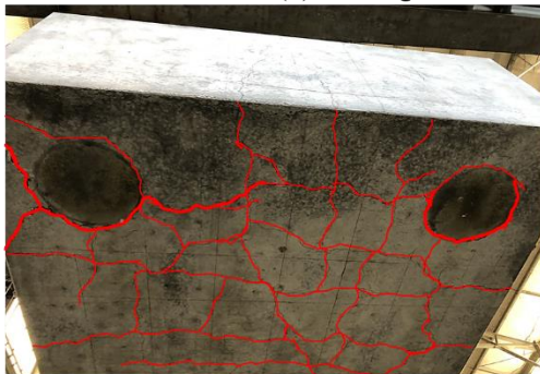
(b) Damage near support side
