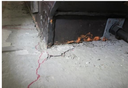
(c) Damage near loading side
