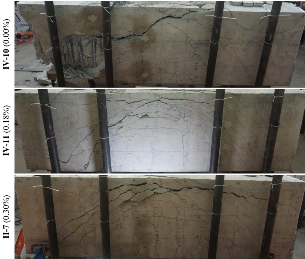
Figure 4.46 Comparison of post-failure conditions on the side faces between specimens: Series IV
