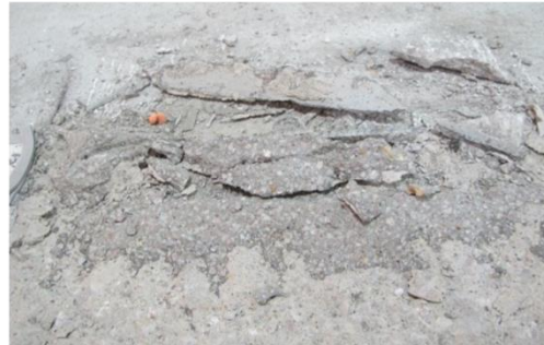
(b) Crushing of column corbel on loading side
