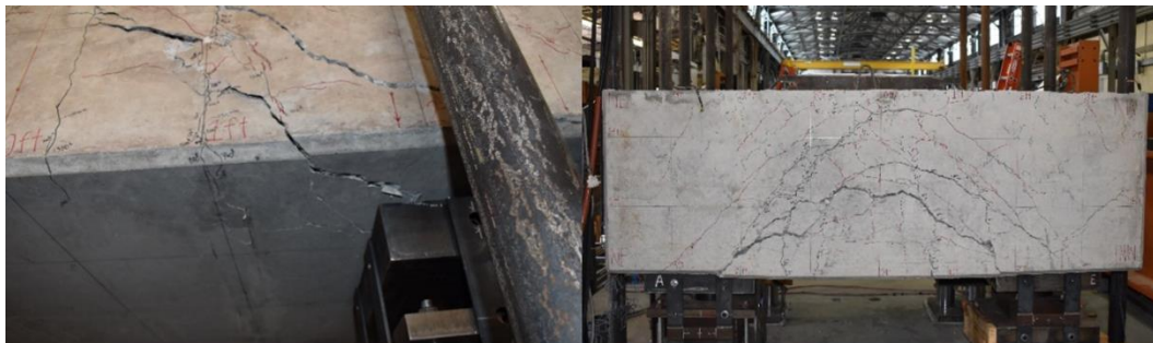
(a) Damage near supports: I-2
