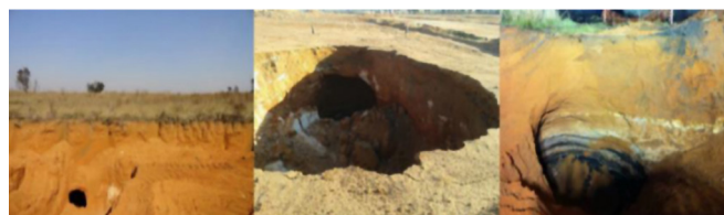
Figure 4—Formation and propagation of sinkholes from old workings voids (visited mine)
