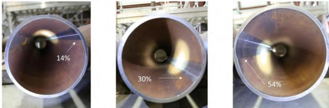
Figure 1. 2 - Sections of worn casing pipes (with percentage of wall thickness removed) [51]
