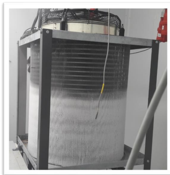
Figure 3.6 Frost build-up process over evaporator
