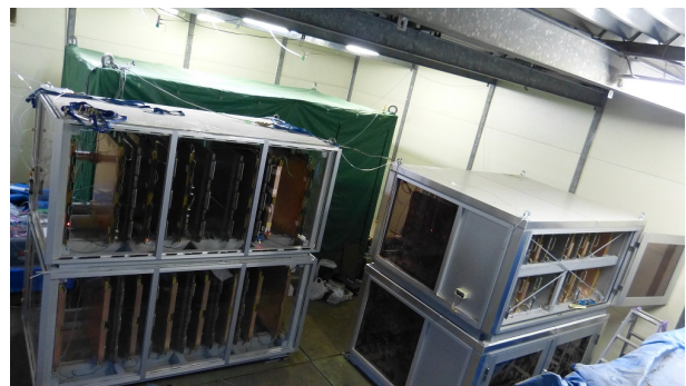
Figure 4. Photo where 2+2 MMOS-es are visible within their container boxes, all inside the simple building of SMO on the hillside of Sakurajima.
