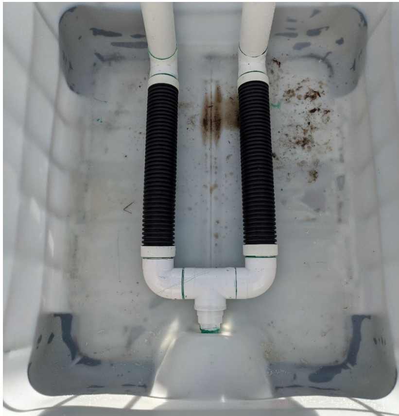
Figure 16: Subsurface collection and drainage system
