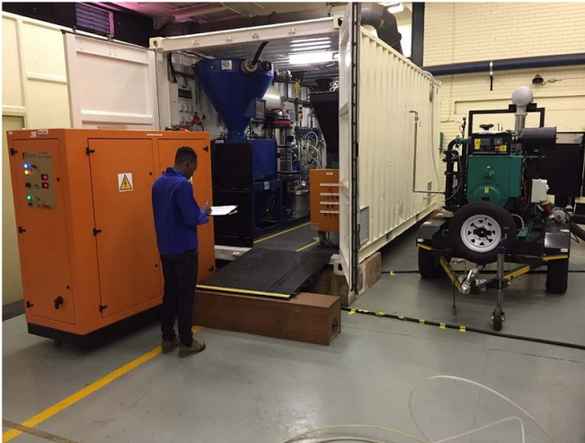
Figure 29. Containerized plasma waste to energy system.
