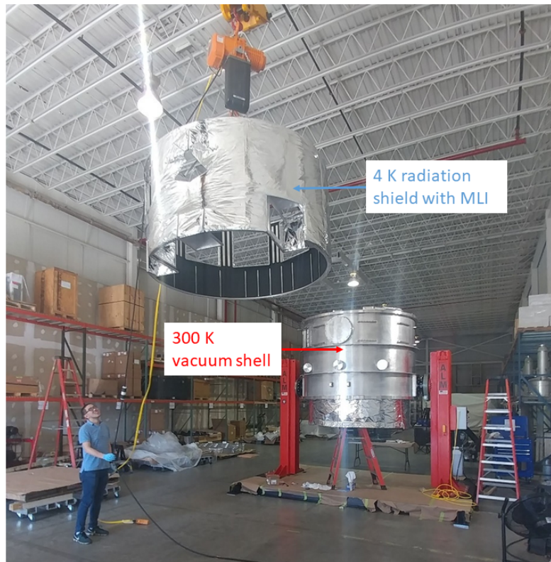
Figure 2.12: This picture shows the 4 K shield right before it is installed in the cryostat. Although the radiative thermal loading from 40 K to 4 K is low, we still wrapped the 4 K shield with 20 layers of MLI, in case excess amount of stray light from 300 K hits the 4 K shield. The black paint on the interior wall of the 4 K shield is also visible in this picture.
